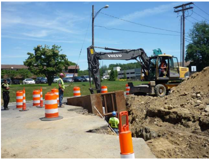
Our experienced construction administration staff play an active role throughout design, construction, and project close-out. Pictured above: Tighe & Bond providing construction observation services for drainage improvements at Bridgeport Hospital.
