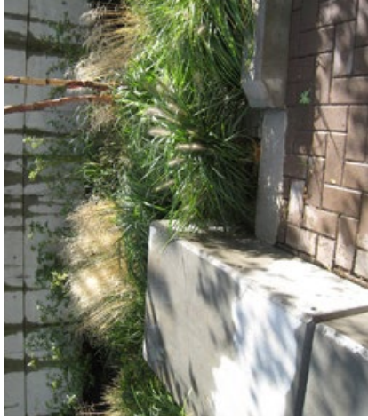
Slotted curb allows water to flow into planting bed
